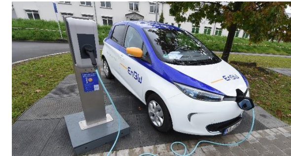
E-mobility charging infrastructure
